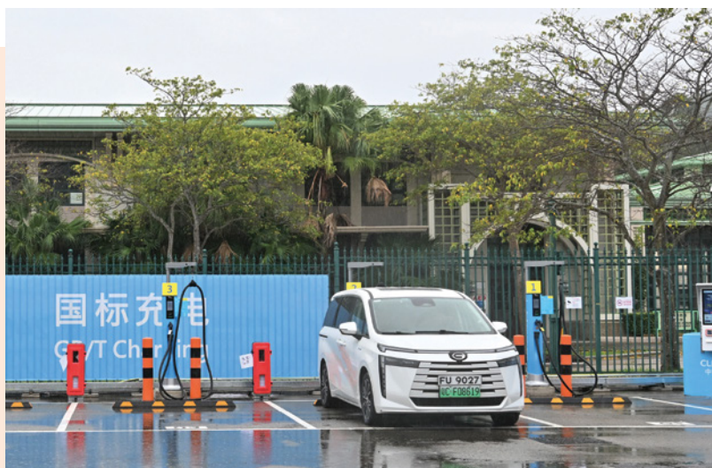
Lantau Charging Station
